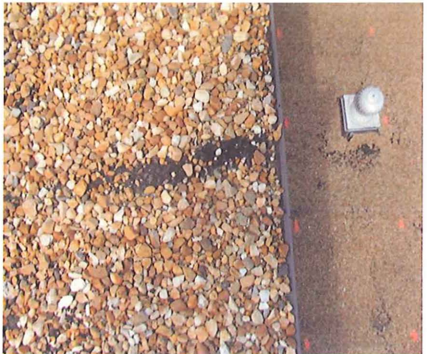
18. Deficiency #7 - Suspect gravel stop stripping
