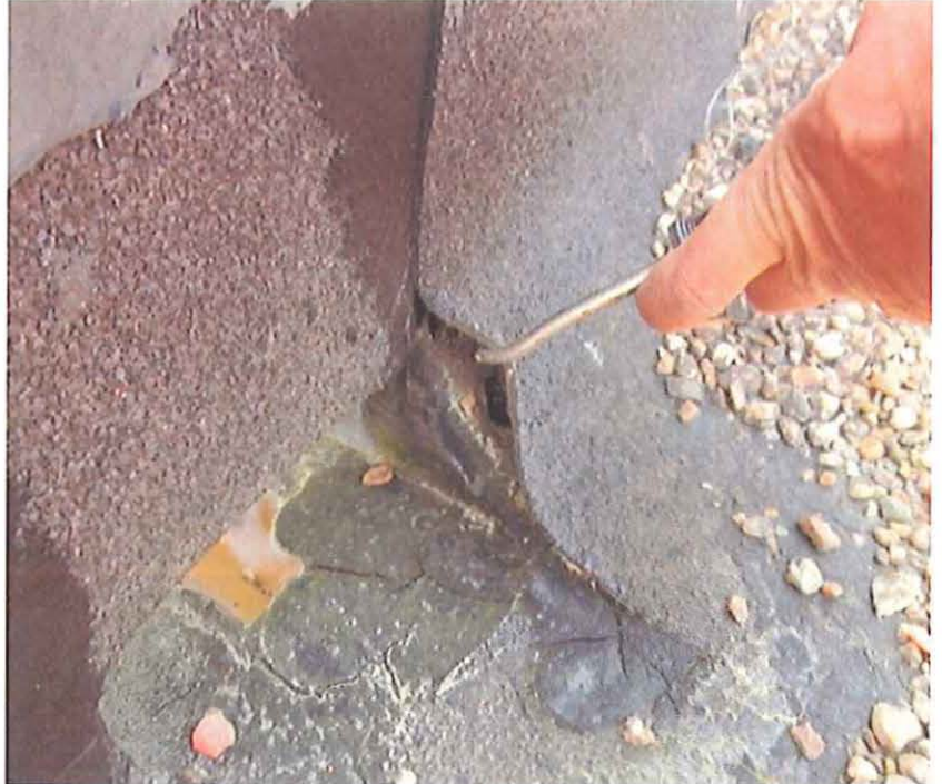
13. Deficiency #4 - Open condition at wall flashing lap
