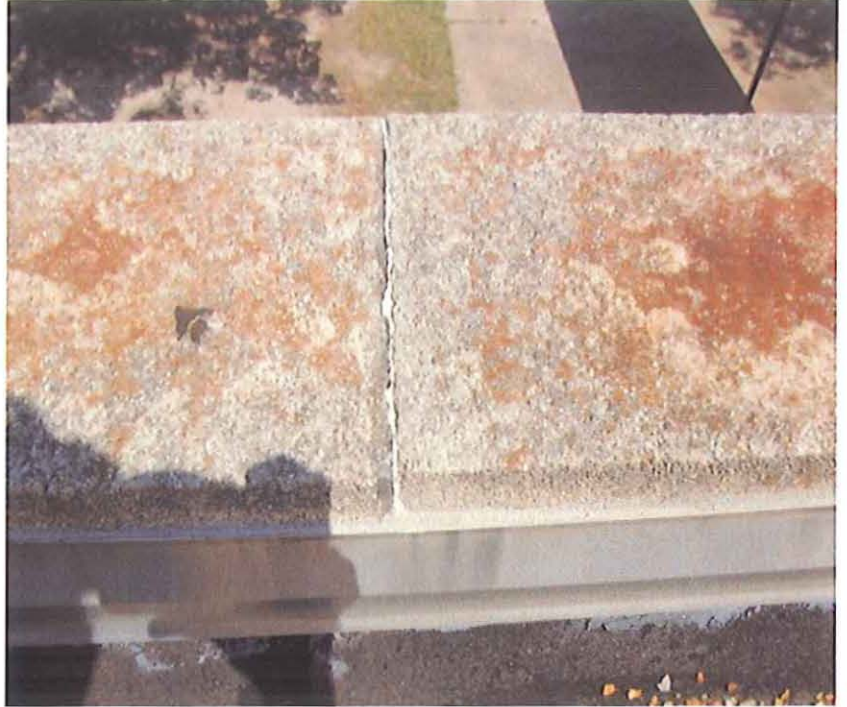
9. Deficiency #2 - Open coping joint
