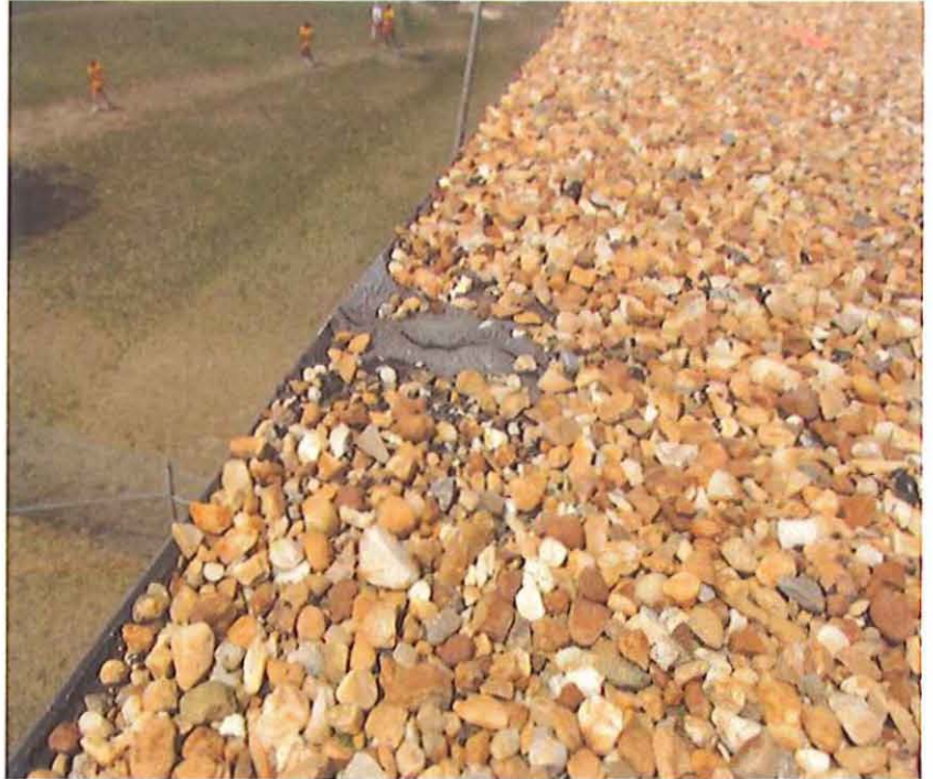
17. Deficiency #7 - Suspect gravel stop stripping
