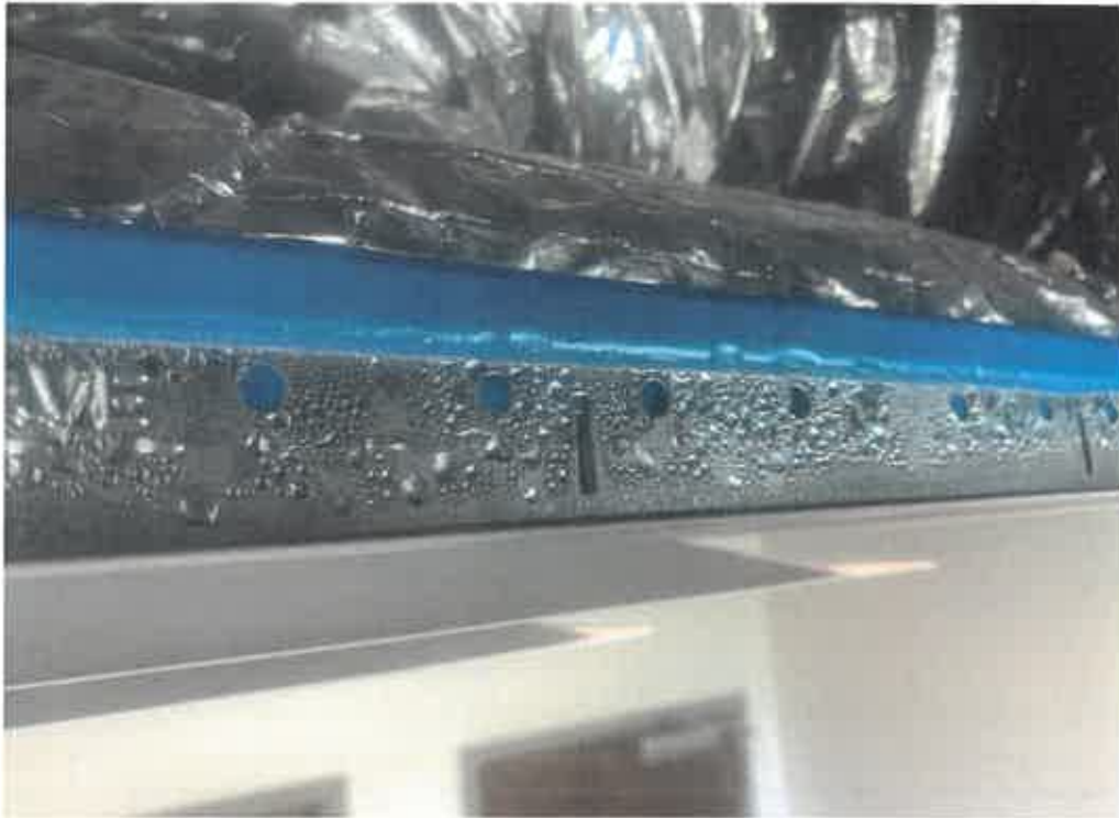
Photo 7: Condensation on the ceiling track near the diffusers
