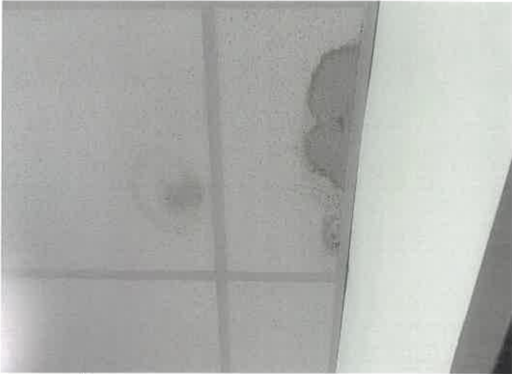
Photo 5: Various stained tile throughout
