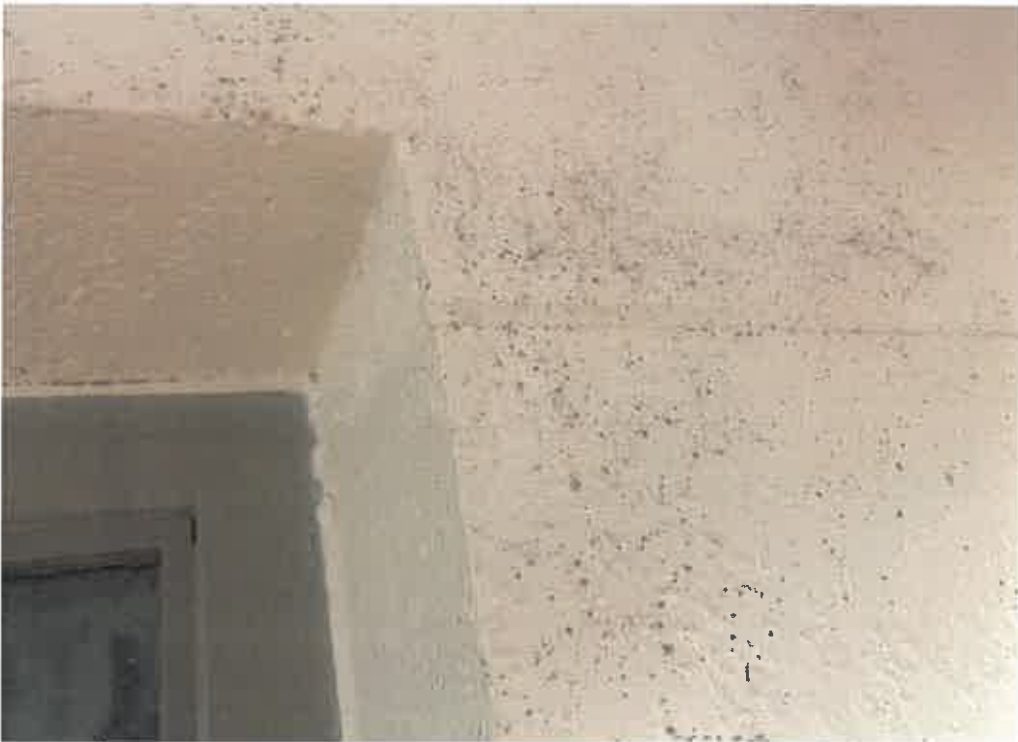
Photo 8: Visible mold on the CMU in the lounge area
