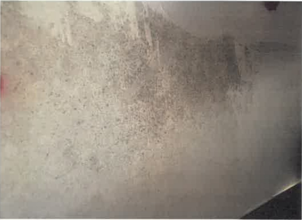
Photo 6: Visible mold on the wallboard above the suspected ceiling in the office
