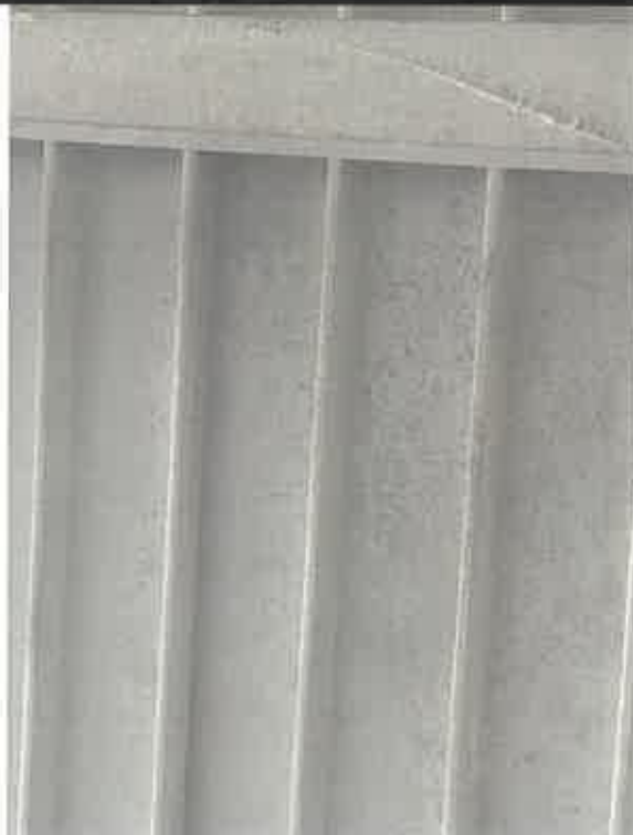
Photo 12: Suspect mold on the bottom of the roof deck in the at room
