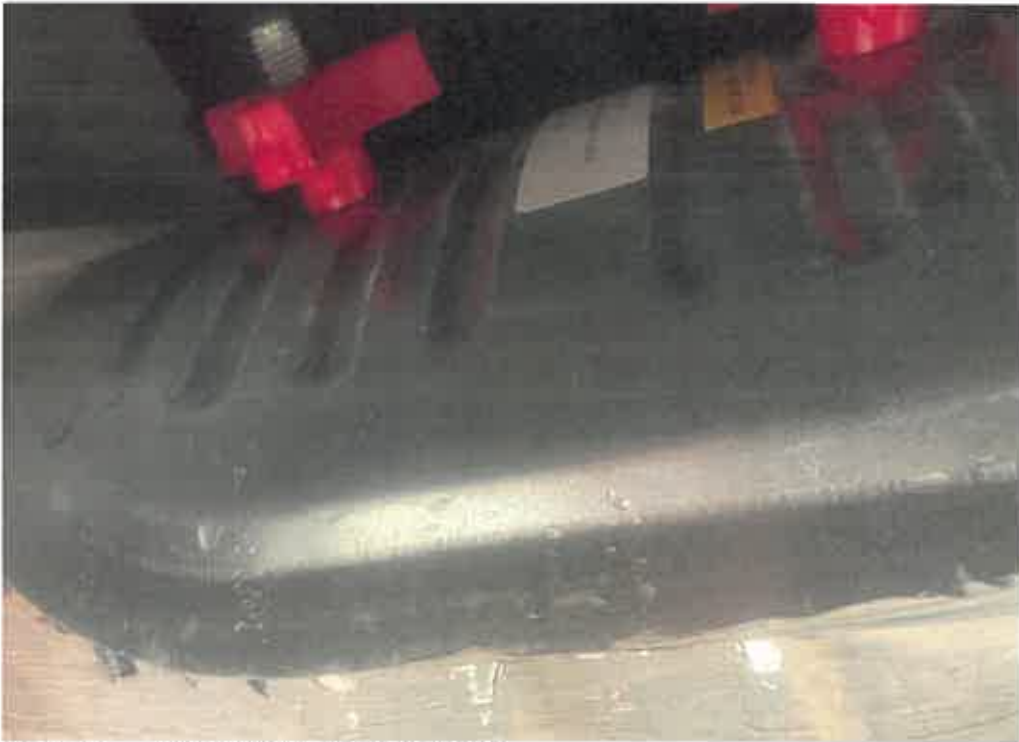
Photo 4: Condensation on the metal ductwork access doors
