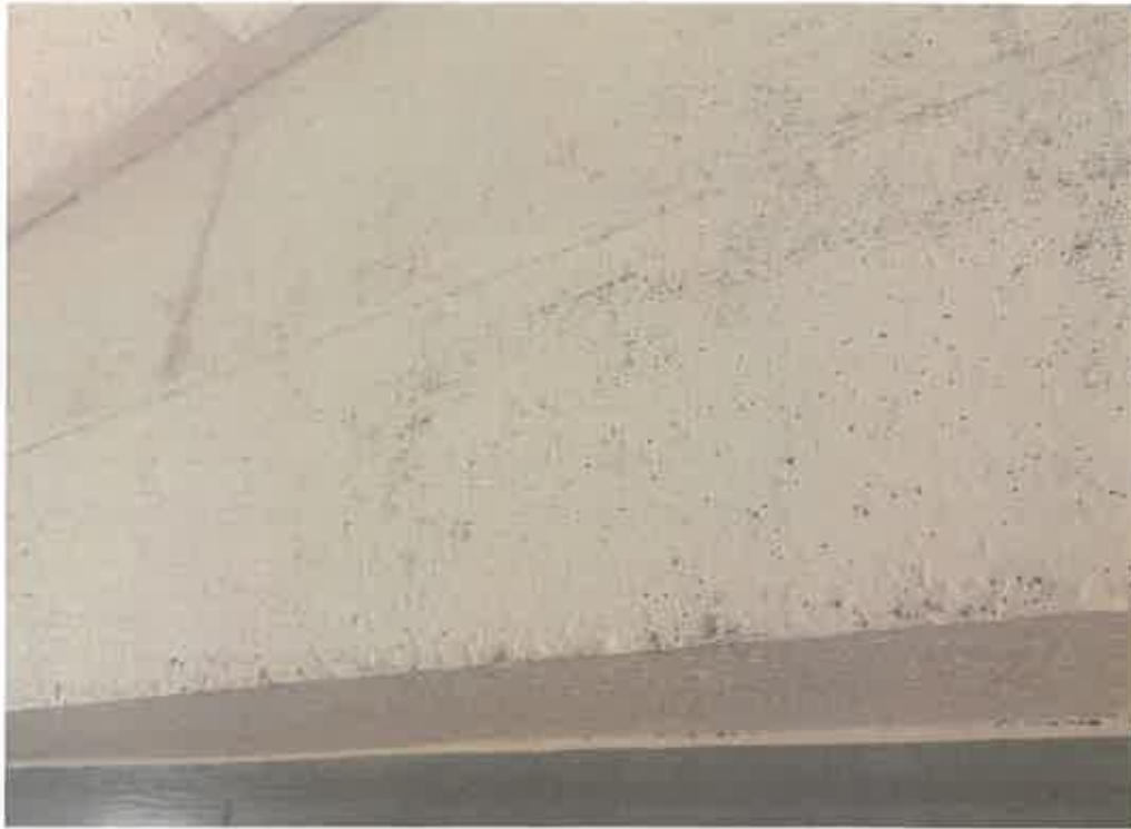
Photo 9: Visible mold on CMU in the lounge area
